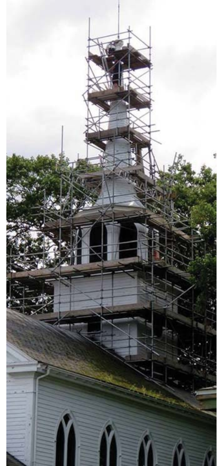
Photo: Steeple restoration is well underway at St. Luke's Anglican Church in Annapolis Royal.
