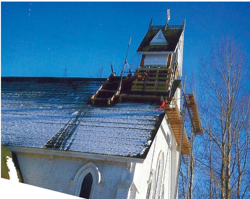
New belfry getting installed on St John the Baptist Anglican Church in Maitland, Hants County.
